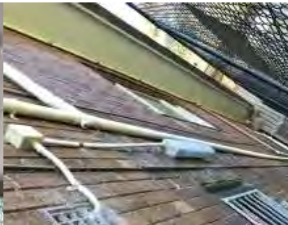
Figure 6 – Tennis Club external lighting
