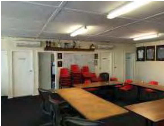
Fig 21 – Soccer Club internal lighting
