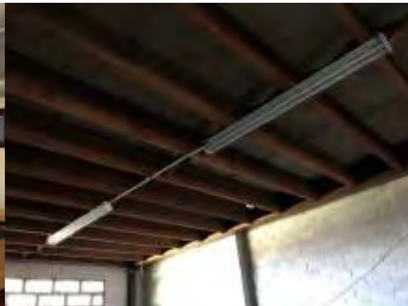
Fig 22 – Soccer Club internal lighting
