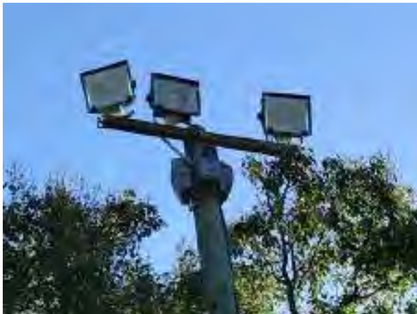
Fig 7 – North Rocks Park Floodlighting
