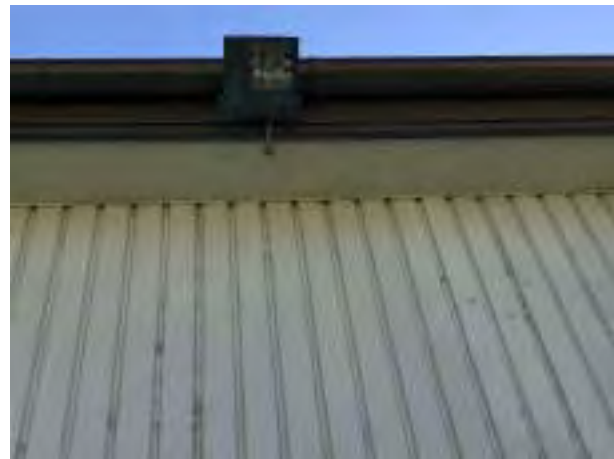
Fig 20 – Community Centre external breakout area lighting
