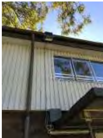
Fig 19 – Community Centre external breakout area lighting
