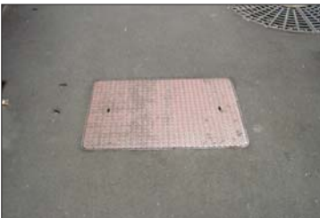
Steel pit cover
