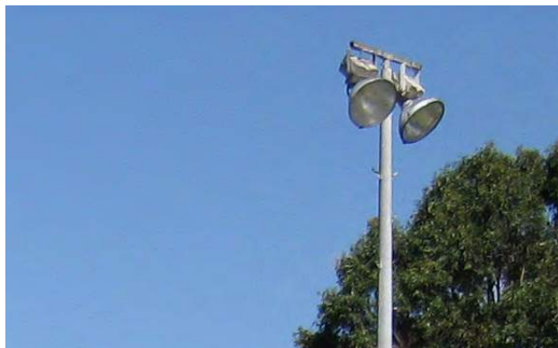
Sports Lighting At Tennis Courts - GKR
