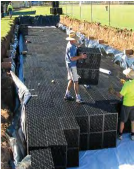
Underground stormwater detention and reuse tanks
