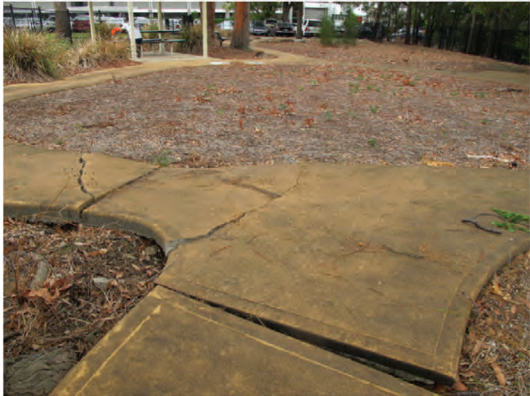
P2: Damaged surface. Unmaintained planter beds
