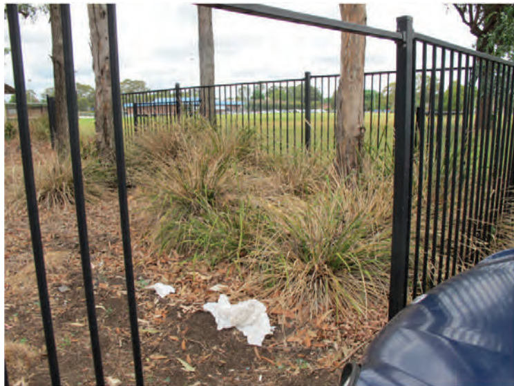
F5: Missing pickets
