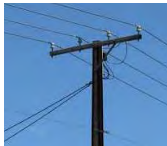
Existing overhead cables. Source: sa.gov.au
