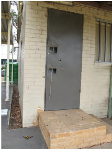
A2: Damaged Door
