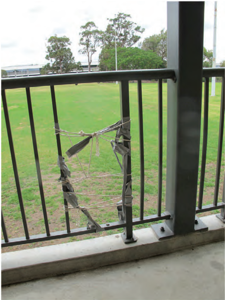
A1: Damaged balustrade
