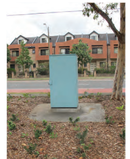
Traffic light control box near Victoria Rd
