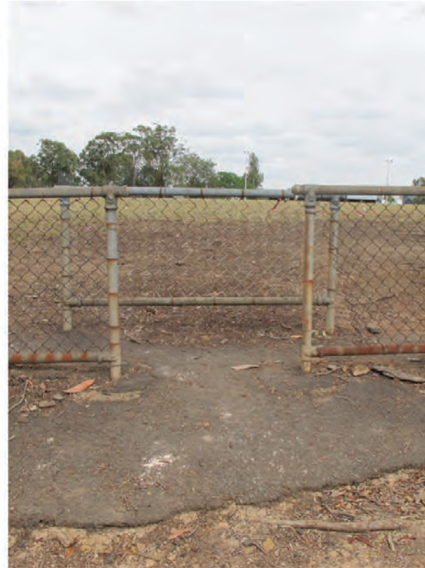
PE5: Stepped fence. Old fence. Poor surface
