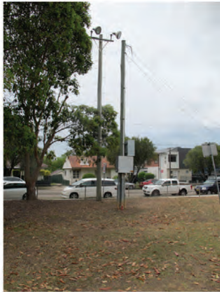
L11: 2 x lanterns. Timber post
