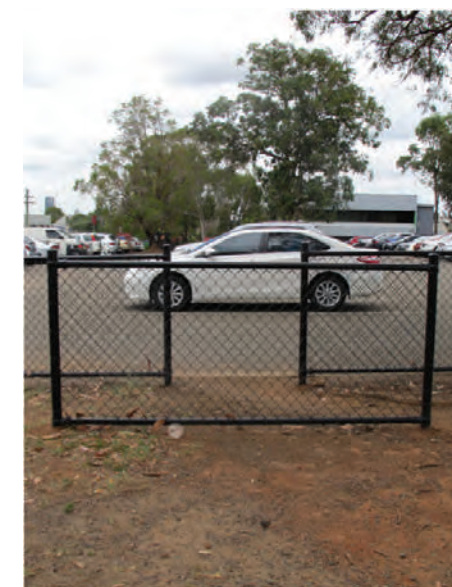
PE8: Stepped fence. New fence. Poor surface
