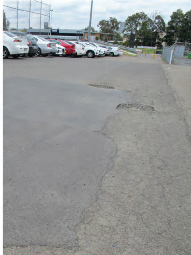
CP1: Patched bitumen with large potholes
