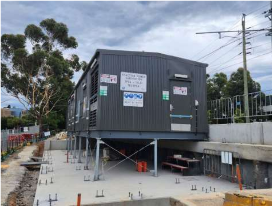
The substation will convert grid electricity to provide power for the operation of the light rail vehicles.
