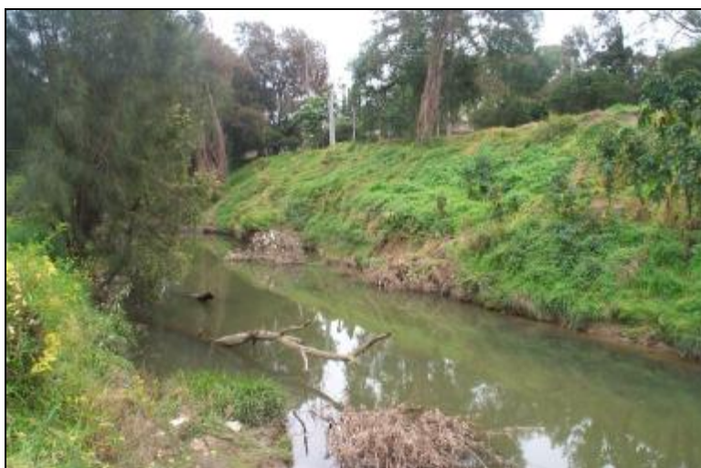
Plate 4 Concave Bank Slumping at Site of Proposed Bank Protection Works
